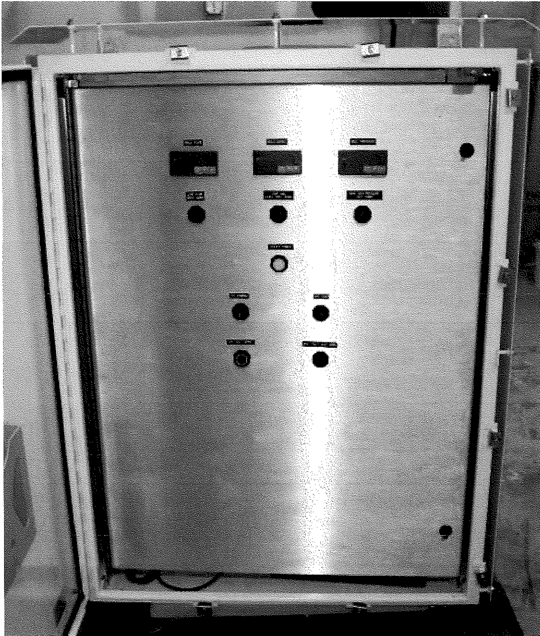
NRO Well Field – Pump Control Panel Door
