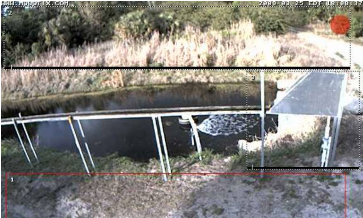
Picture 1. Powell Creek Influent, Surger and Flowway (picture taken via security camera)
