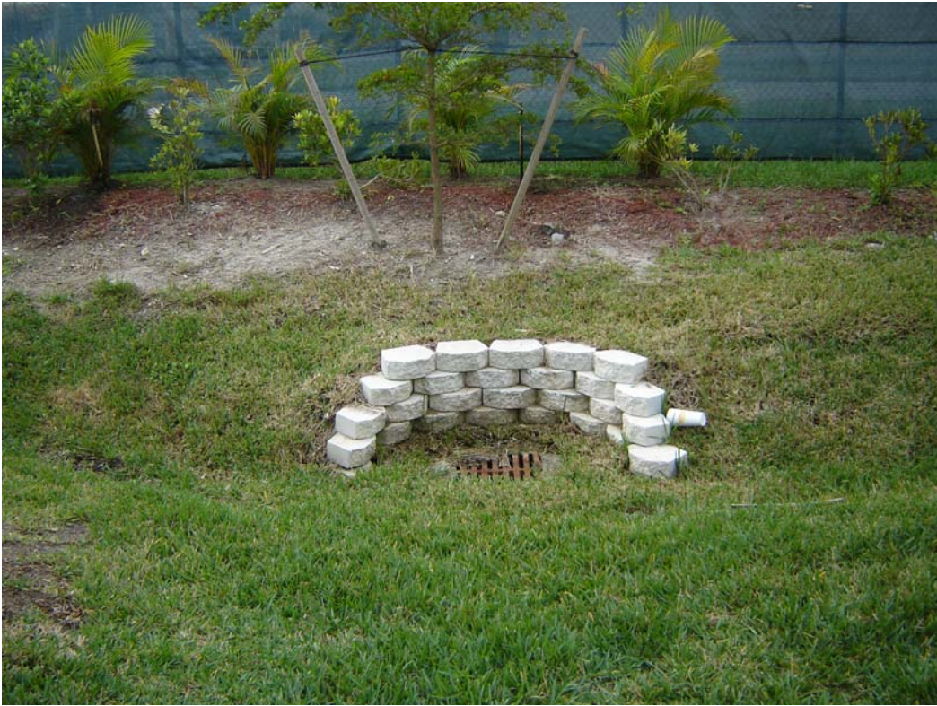
Laguna Lakes – Yard Drain
