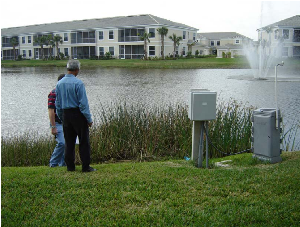
Laguna Lakes – Fountain Aeration
