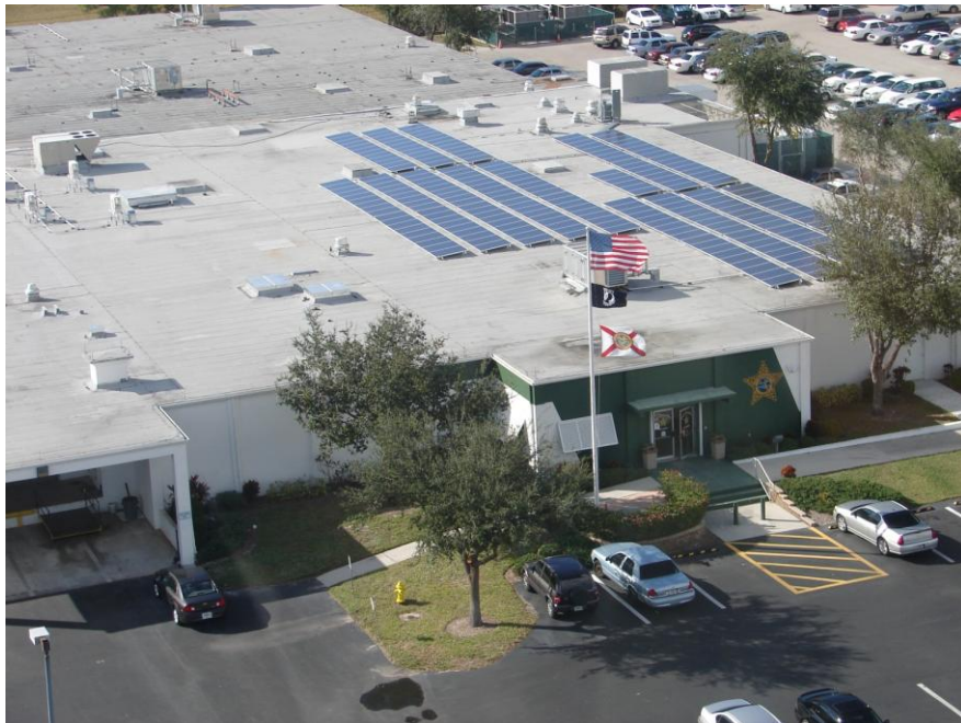
New photovoltaic array at Public Safety on 6 Mile Cypress
