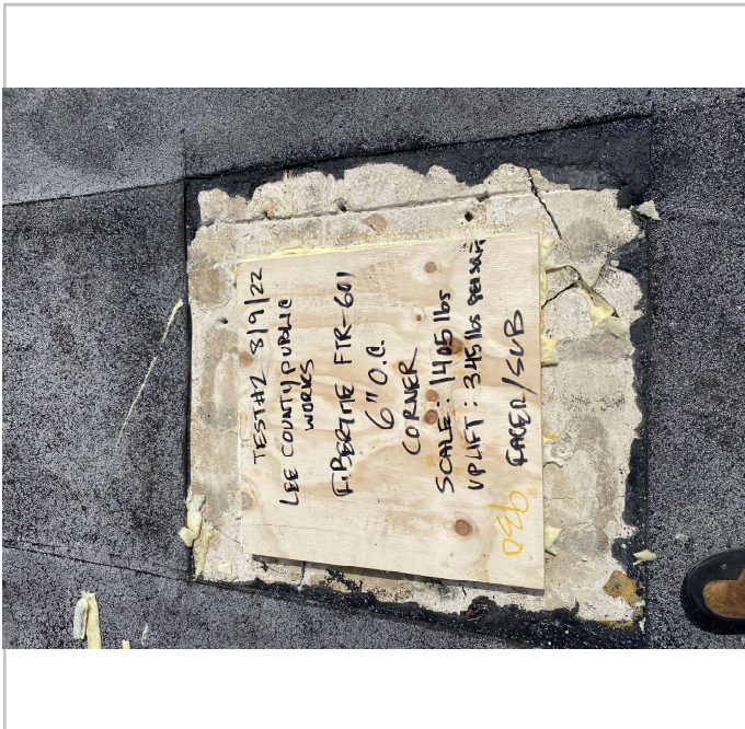
TEST #2 6" O.C. CORNER
