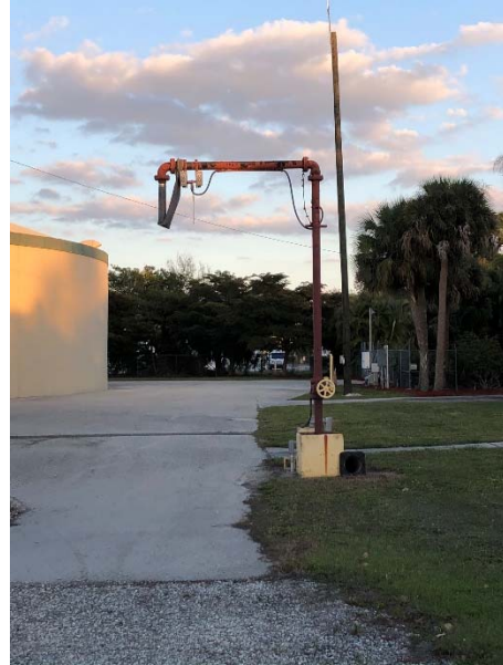
Photo 4. Truck Loading Arm (D16)
