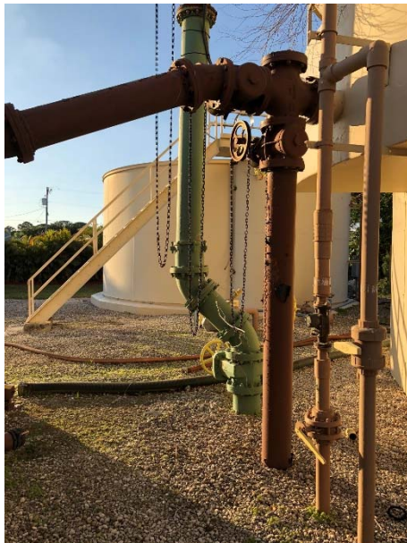
Photo 1. Brown Pipe with LBP rfont of Clarifier
