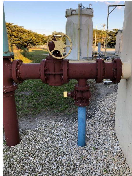
Photo 2. Brown LBP Pipe rear of Clarifier
