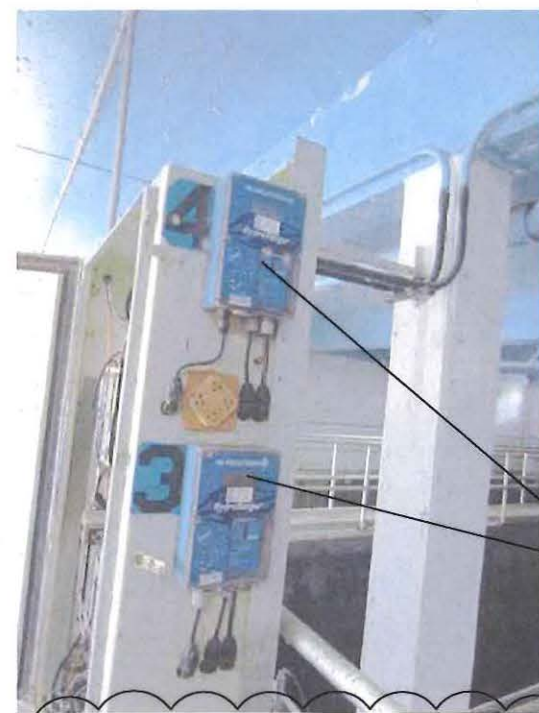
△ FIGURE 3: EXISTING FILTER LEVEL TRANSMITTERS (FILTERS 3 & 4)
