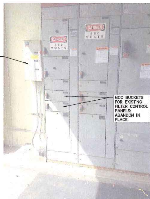
PHOTO 8 MTS FOR PANEL LC AND PARTIAL VIEW OF MCC 4A SCALE: NTS
