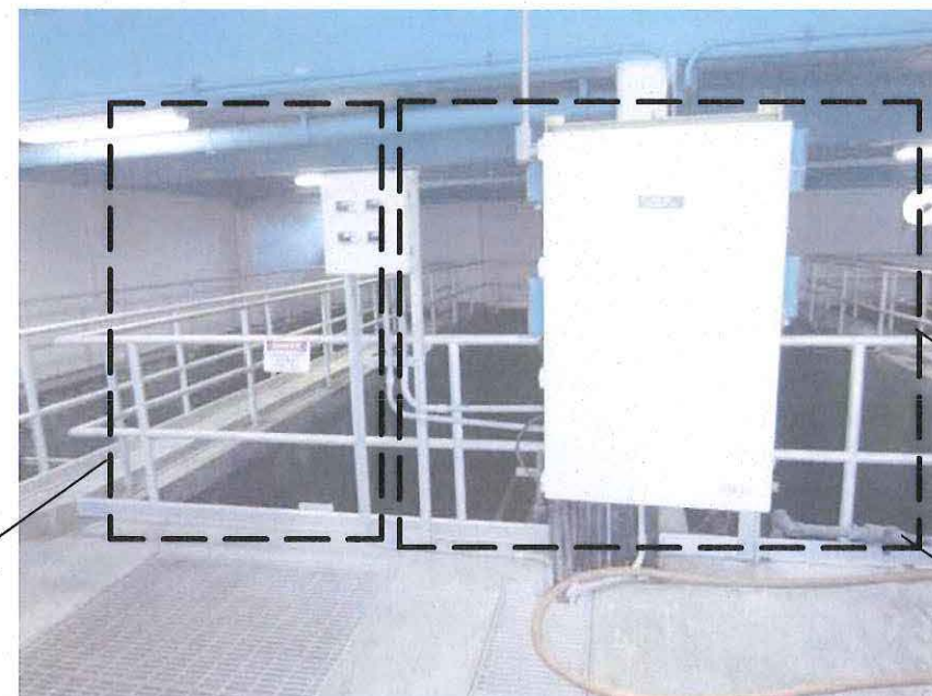
FILTER LEVEL TRANSMITTER PANEL RACK & FILTER PLC PANEL LOCATION
