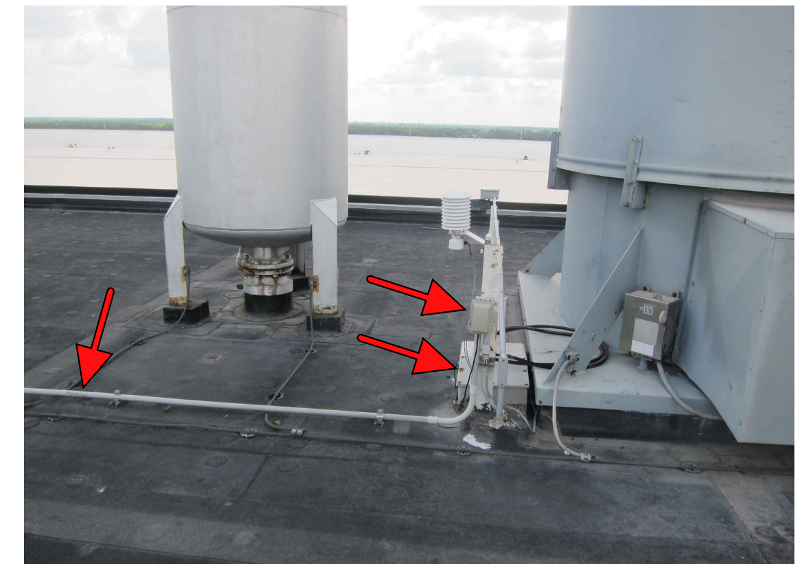
16 BOILER #1 & #2: ELECTRICAL BOX / OULET AND CONDUIT LINES.
