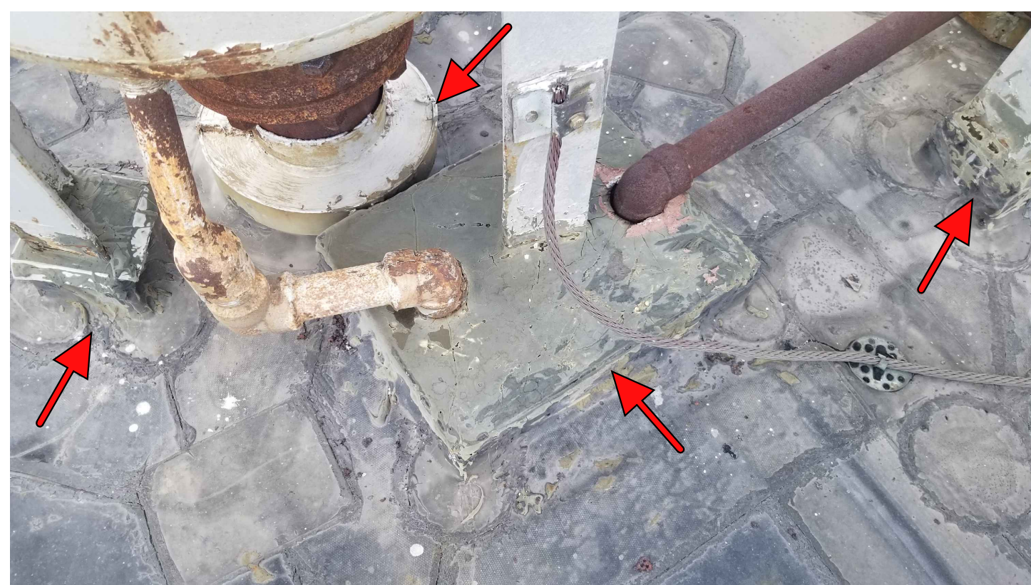
13 BOILER #1 & #2: EXISTING PITCH PAN AND PENETRATIONS.
