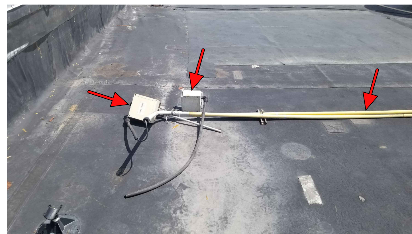
15 BOILER #1 & #2: ABANDONED COMMUNICATION / ELECTRICAL BOX AND CONDUIT LINES.
