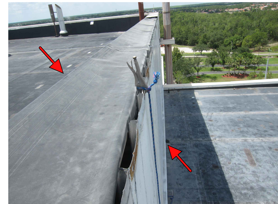
8 BOILER #1 & #2: EXISTING PARAPET WALL AND METAL SIDING PANEL. MISSING COPING CAP.
