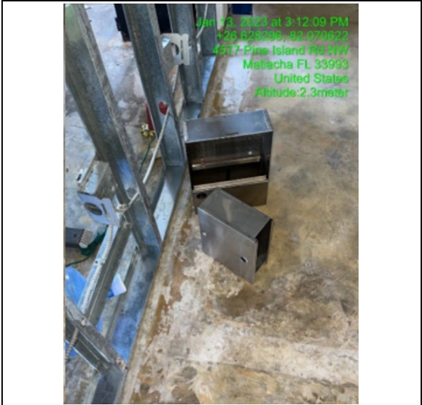
Photo #: N/A Description: Displaced bathroom specialties/accessories
