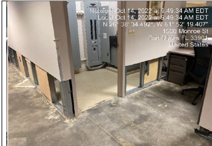
Photo #: 31.01, 31.02, 31.03, 31.04 Description: Electrical Room 111 vinyl composition tile, flooring, drywall, vinyl base, insulation
