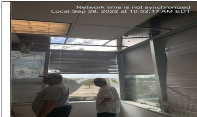
Photo #: 6.07, 6.08, 6.10, 6.11 Description: Double pane glass, foil face fiberglass insulation, and ceiling tiles
