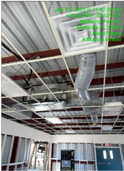
Photo #: 5.01, 5.09, 5.11 Description: Diffuser high performance three cone.
