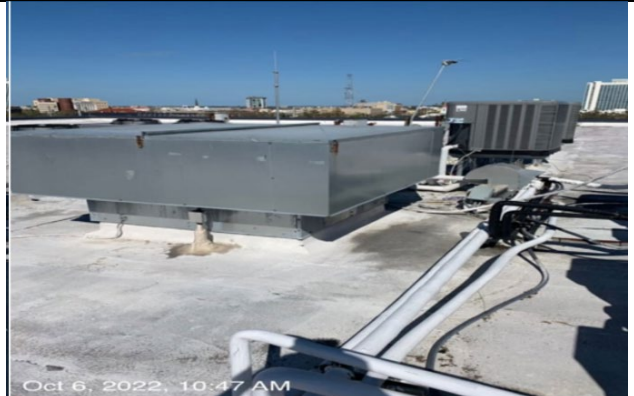
Photo #: 1.06 Description: Supply Connecting pipes
