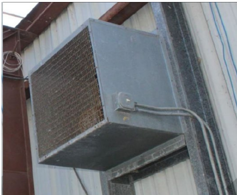
Photo #: 2.11 Description: Ventilation fan with motor rated switch
