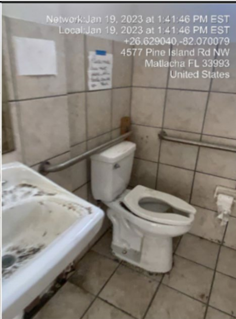
Photo #: 5.09 Description: Restroom tank type toilets
