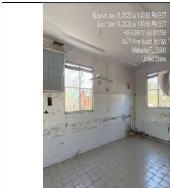
Photo #: 2.04, 2.11, 2.17 Description: Drywall with mold growth, ceiling fan
