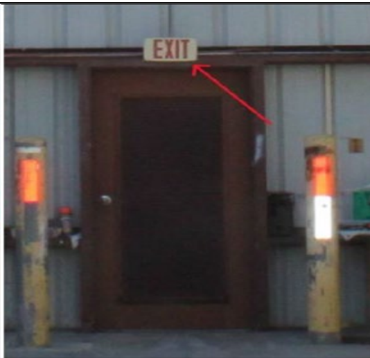
Photo #: 2.03 Description: Thermoplastic exit sign
