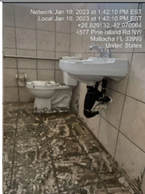
Photo #: 5.03, 5.09 Description: Restroom wall mounted lavatory
