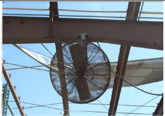
Photo #: 2.10 Description: Cage circulating fan
