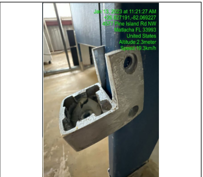
Photo #: 3.09 Description: Rusting interior metal doors.
