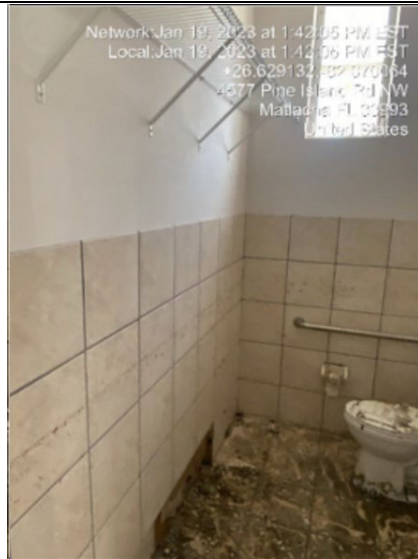
Photo #: 5.03, 5.02 Description: Restroom tile high-mark
