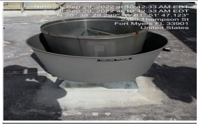
Photo #: 1.05 Description: Halon Purge cap
