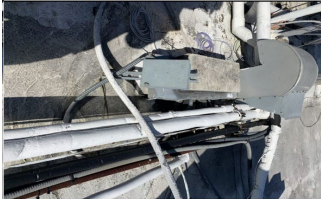
Photo #: 1.06 Description: Supply connecting pipes
