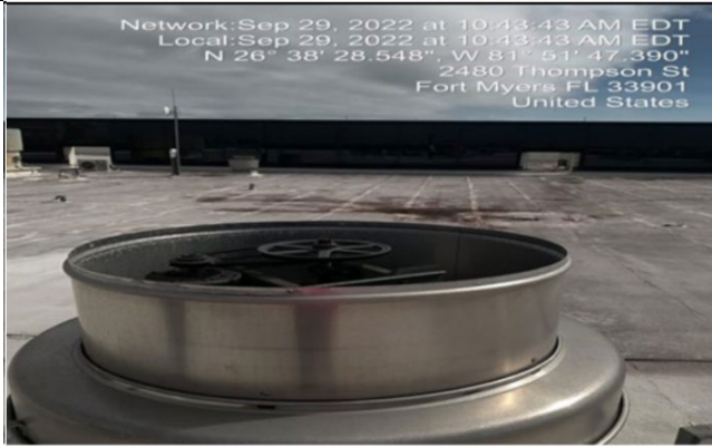
Photo #: 1.04 Description: Exhaust fan cap
