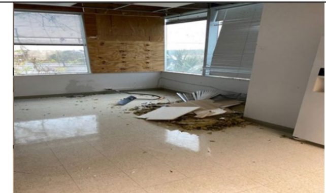
Photo #: 6.04, 6.08, 6.10, 6.11 Description: Debris (Insulation, ceiling tiles, insulation board, glass)
