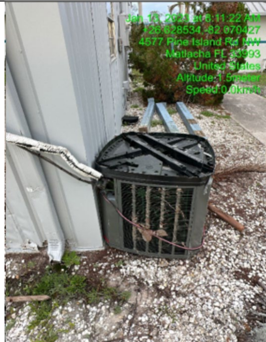
Photo #: 4.01 Description: Refrigerant lines dislodged by storm surge.
