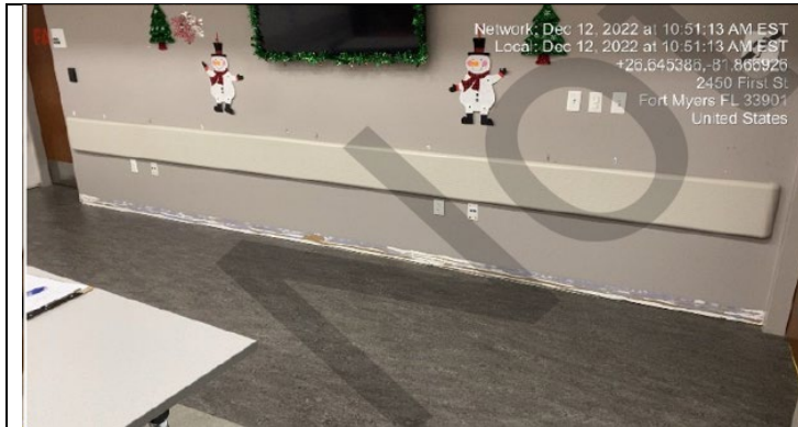
Photo #: 23.01 Description: Room 133 Storytime/MTG Room baseboard
