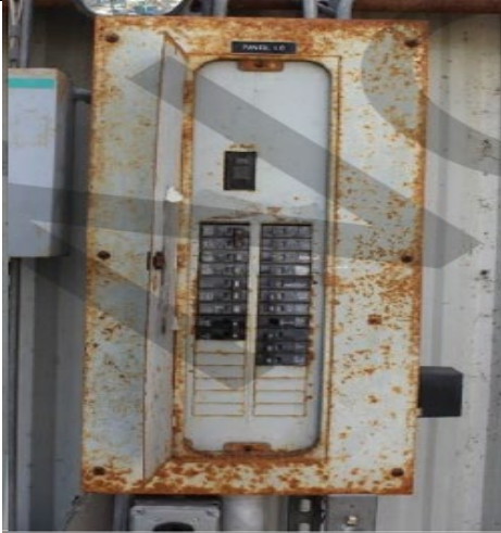
Photo #: 2.13 , 2.14 ,2.15, 2.16, 2.17, 2.18 Description: Siemens, 3-phase, copper bus, 100 Amp, main breaker type, NEMA 1 load center
