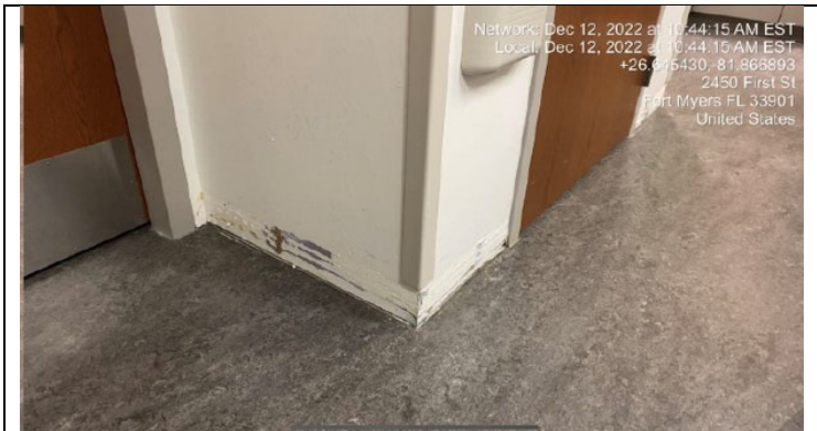
Photo #: 21.01 Description: Room 132 YA/YS Workroom baseboard
