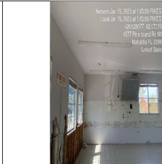
Photo #: 2.04, 2.06 Description: Drywall with mold growth, high-water on the wall
