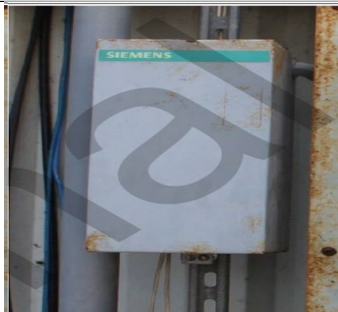
Photo #: 2.12 Description: Siemens lighting contactor
