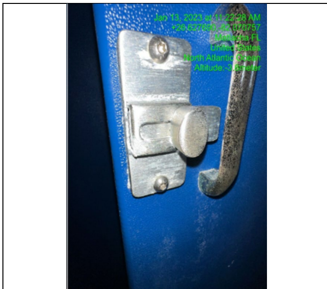
Photo #: 3.09 Description: Rusting interior metal doors.
