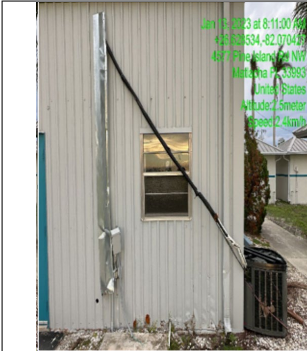
Photo #: 4.01, 4.02, 4.04 Description: Electrical conduit/refrigerant lines dislodged
