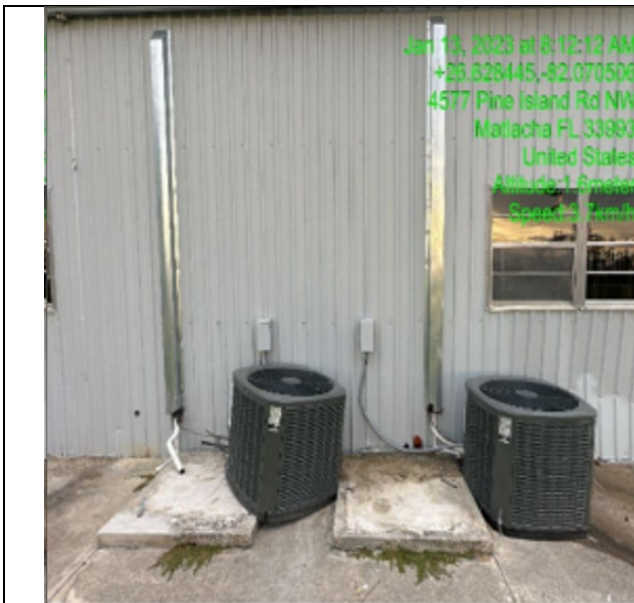
Photo #: 4.01, 4.03, 4.04 Description: HVAC Condensing Units dislodged from Pad
