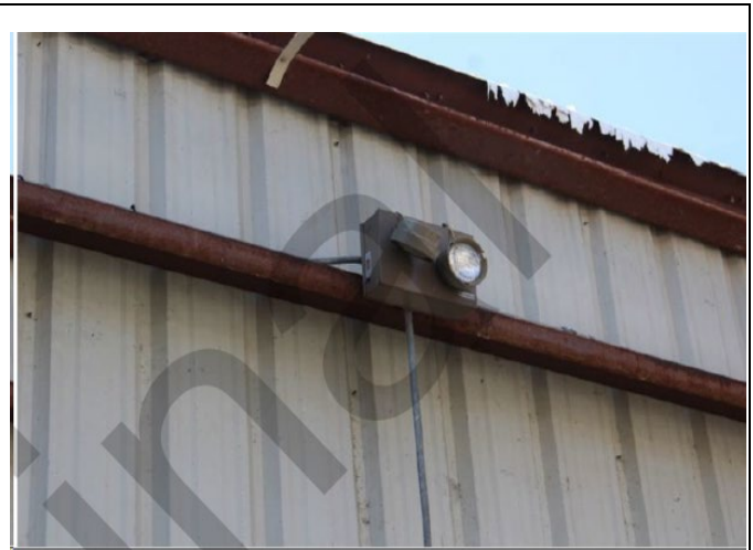
Photo #: 2.04 Description: Lithonia, steel bodied, twin lamp emergency light
