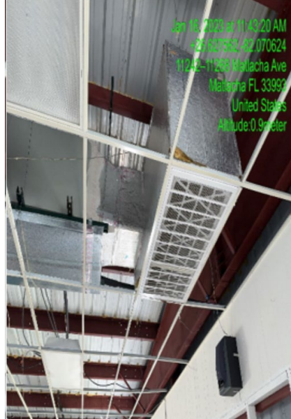
Photo #: 5.12 Description: Return panel steel perforated.
