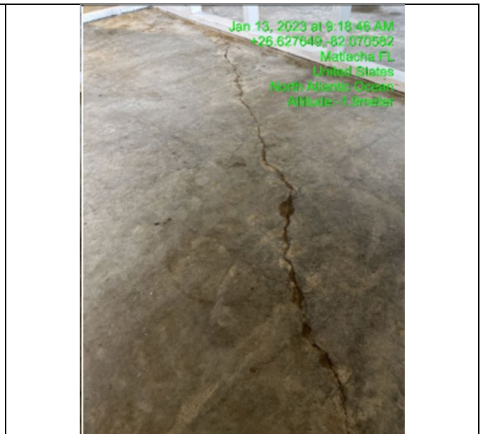
Photo #: 3.07 Description: Flooring vinyl wood grain removed/cracks
