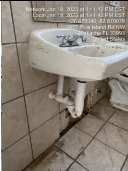
Photo #: 5.03 Description: Restroom plumbing fixtures with close-up high-water mark on side of sink
