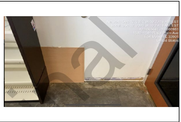
Photo #: 18.03, 18.04 Description: Room 128 Young Adult baseboard, drywall
