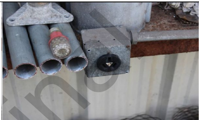
Photo #: 2.08 Description: R10-50 receptacle
