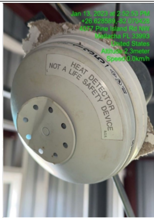
Photo #: 12.02 Description: Displaced heat detector.
