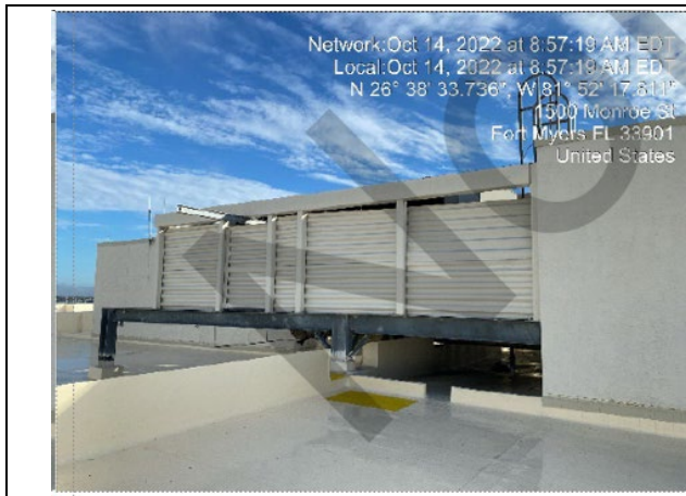
Photo #: Roof 1.06 Description: Chiller Plant wind guard horizontal corrugate metal windscreen
