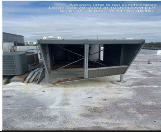
Photo #: 1.03 Description: Exhaust Fan 2
