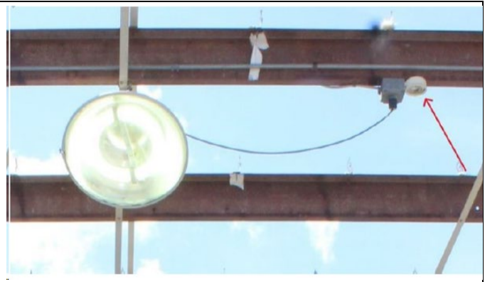
Photo #: 2.02 Description: Light Fixture motion sensors
