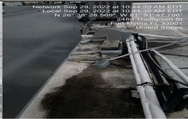
Photo #: 1.06 Description: Supply Connecting pipe
