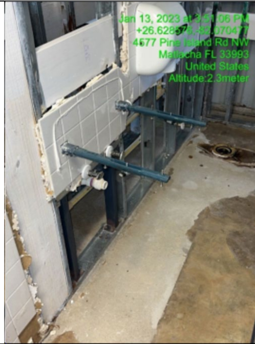
Photo #: 8.02, 8.04, 8.05 Description: Plumbing fixtures.
