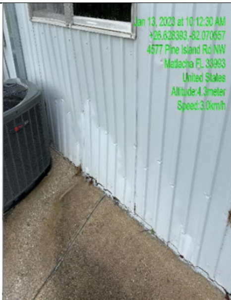
Photo #: 4.01 Description: Damaged exterior HVAC Condensing Unit.
