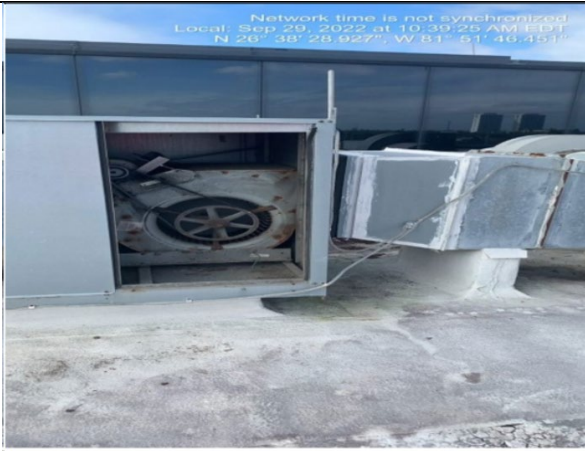
Photo #: 1.03 Description: Exhaust Fan 2
