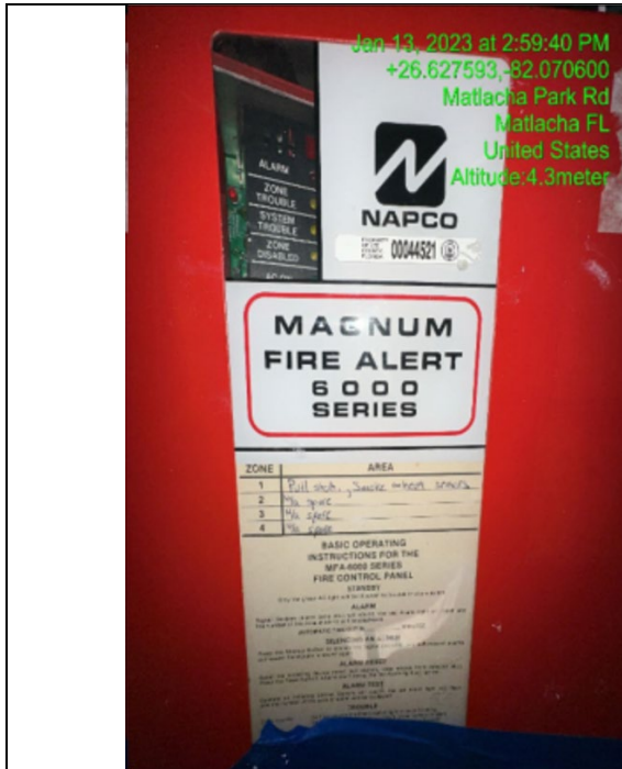
Photo #: 12.01 Description: Fire alarm panel location.
