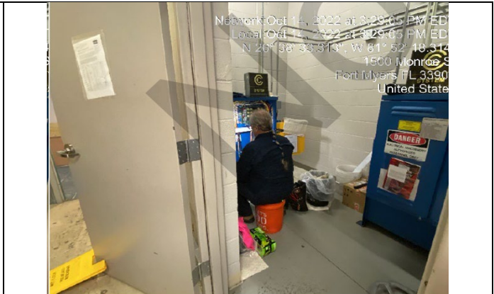
Photo #: 13.01 Description: Elevator equipment room 102 concrete floor, hydraulic system
