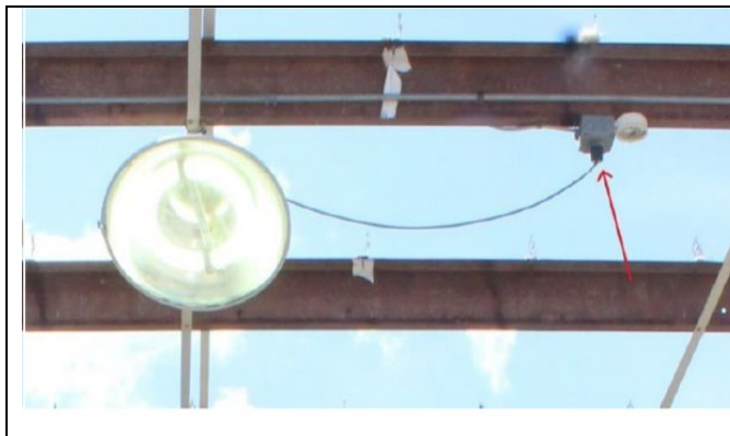
Photo #: 2.07 Description: 20 Amp, 120 Volt, Specification grade twist lock receptacles
