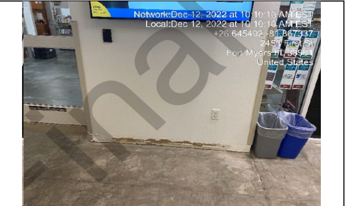
Photo #: 1.02 Description: Rooms 101/103 Lobby baseboard
