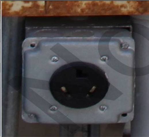
Photo #: 2.09 Description: R10-30 receptacle
