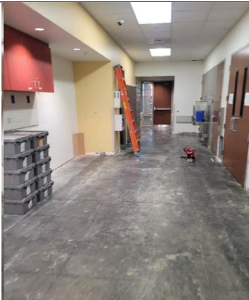
Photo #: 12.01, 12.02, 12.03 Description: Rooms 120/114 Receiving (Corridor) carpet tile, baseboard, drywall
