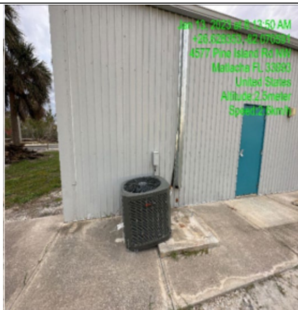
Photo #: 4.01, 4.03, 4.04 Description: HVAC Condensing Unit dislodged from Pad
