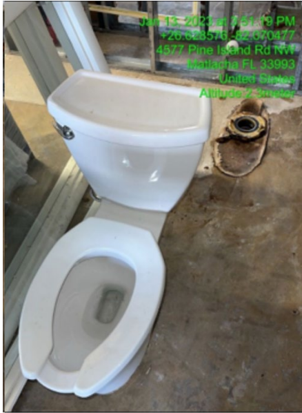
Photo #: 8.01 Description: Plumbing fixtures.
