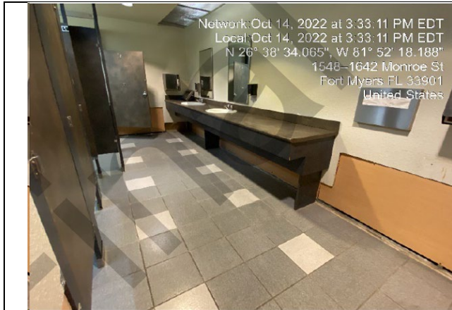
Photo #: 9.01, 9.02, 9.03, 9.04, 9.05 Description: Women's Restroom floor tile, drywall, ceramic wall tile base, insulation
