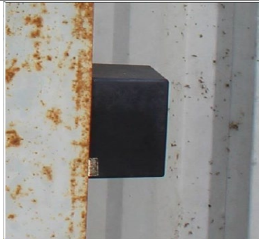
Photo #: 2.19 Description: Nipple mounted surge suppressor
