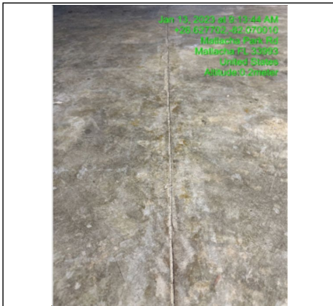
Photo #: 3.07 Description: Flooring vinyl wood grain removed/cracks
