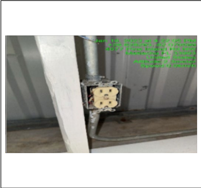
Photo #: 7.04, 7.05, 7.06, 7.08, 7.10 Description: Electrical Outlet, conduit, wiring, all compromised.
