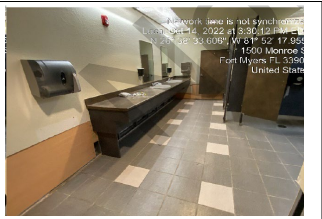
Photo #: 10.01, 10.02, 10.03, 10.04, 10.05 Description: Men's Restroom 108 floor tile, drywall, wall tile, ceramic tile base, insulation
