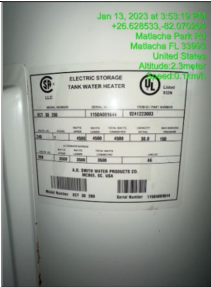
Photo #: 8.09 Description: Plumbing fixtures.
