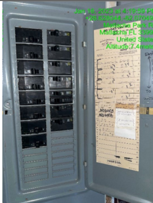
Photo #: 7.01, 7.02 Description: Electrical wall panel.
