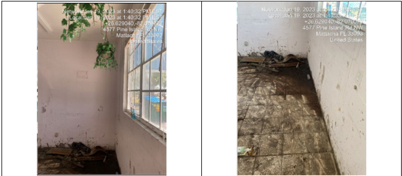
Photo #: 3.01, 3.02, 3.03 Description: Library window with mold growth
