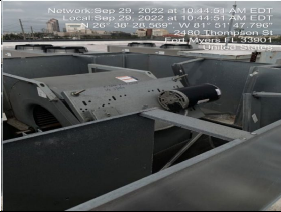
Photo #: 1.02 Description: HVAC supply fan
