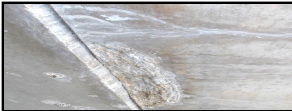
Sample of deck slab spalling
