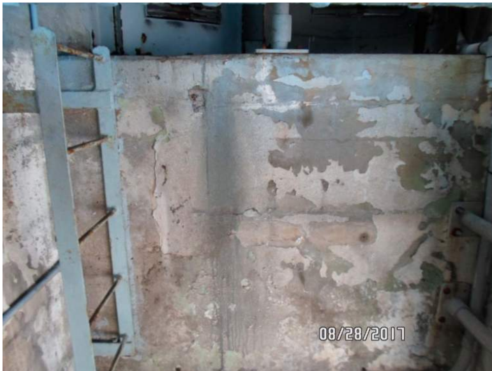
PC-2: Light blue paint with gray undercoating on steel door located on steel wall partition between electrical room and trunnion area
