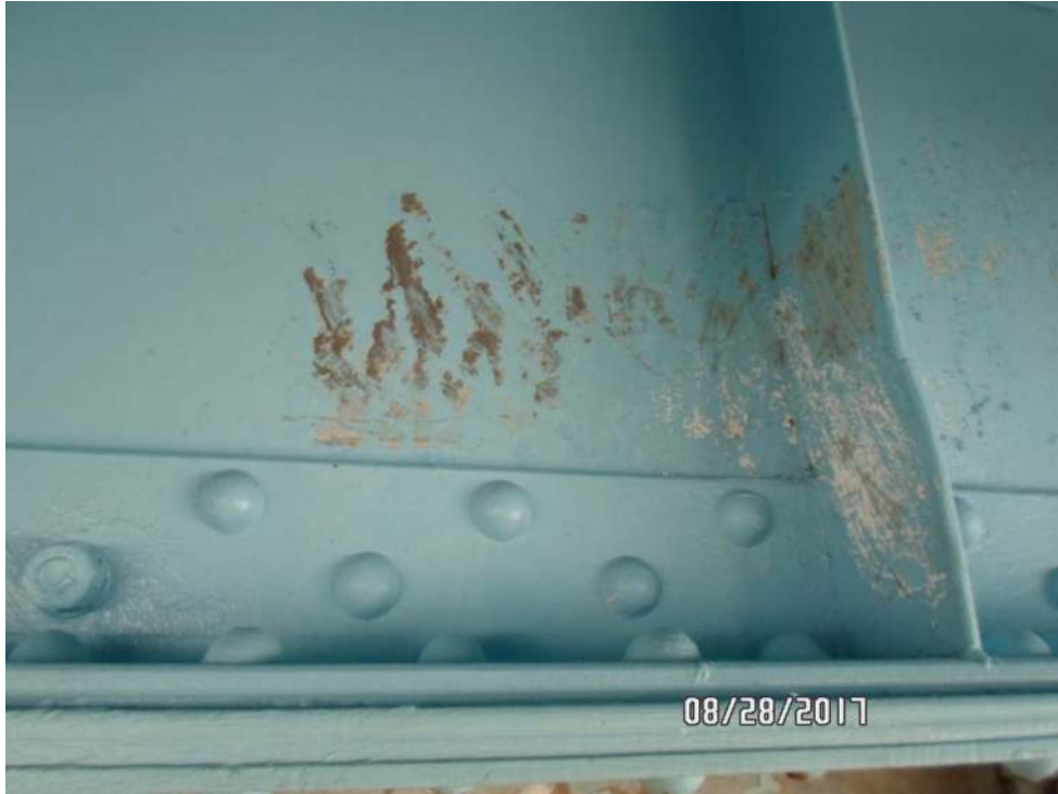
PC-3: Blue paint with white undercoating located on steel bascule girder in trunnion area
