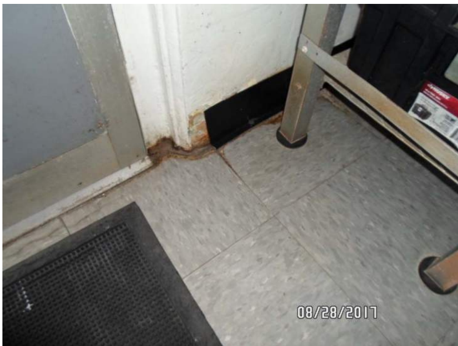
Homogeneous Area #2 (samples 004-006): Black baseboard with light brown mastic; north wall inside tender house
