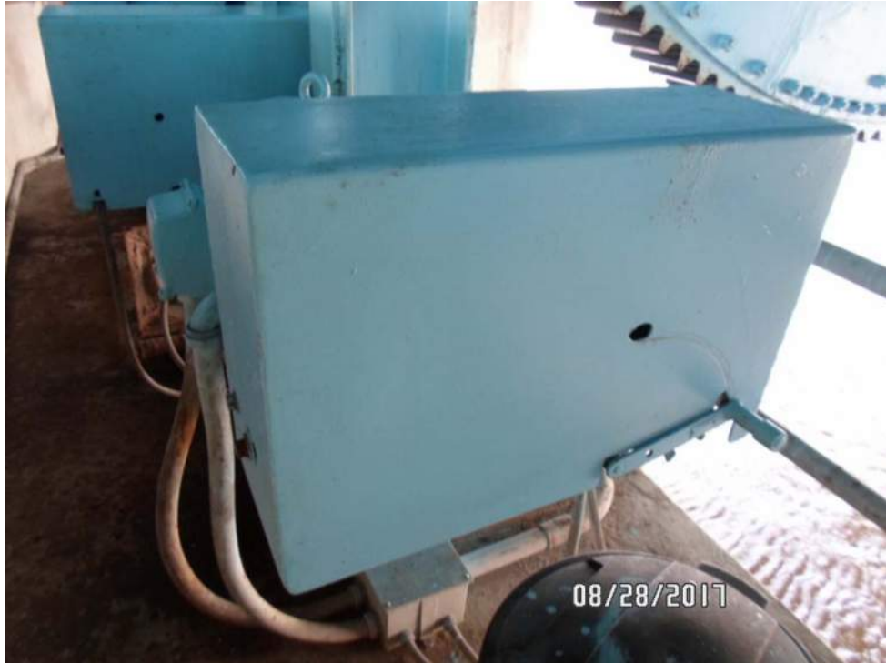
Homogeneous Areas #15 and #16: service brake and emergency brake boxes – east pit
