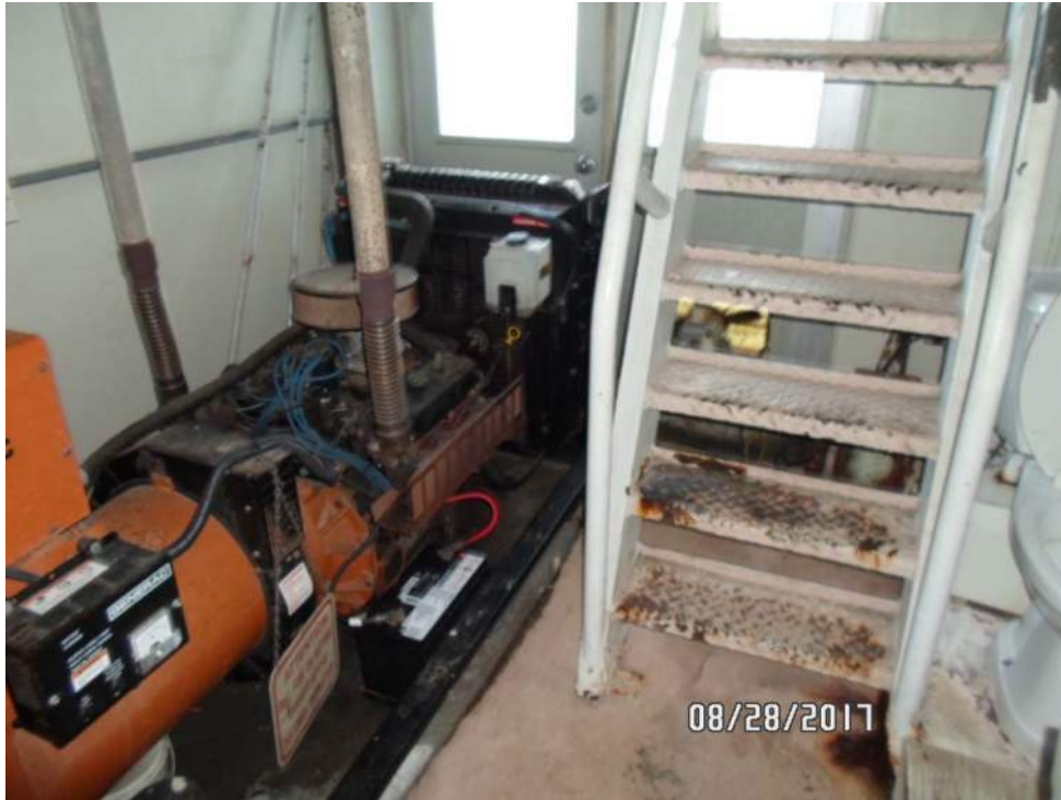
PC-1: White paint with gray undercoating on metal staircase inside electrical room
