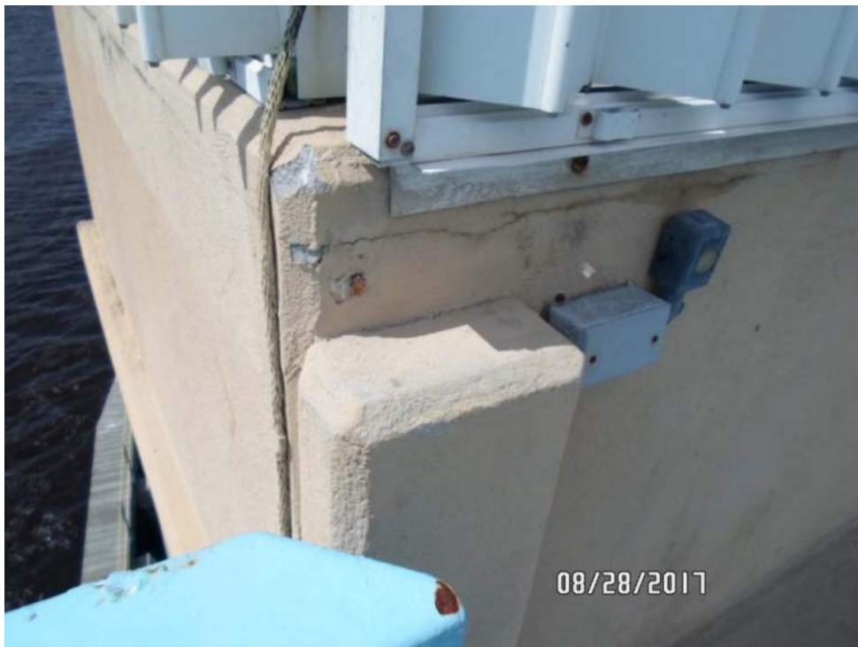
Homogeneous Area #4 (samples 010-011): Gray concrete w/ tan paint, northeast corner of tender house
