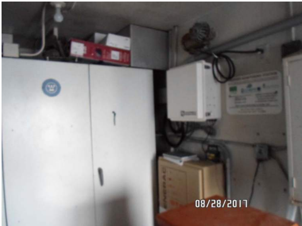
Homogeneous Area #17: Electrical Components – mechanical room
