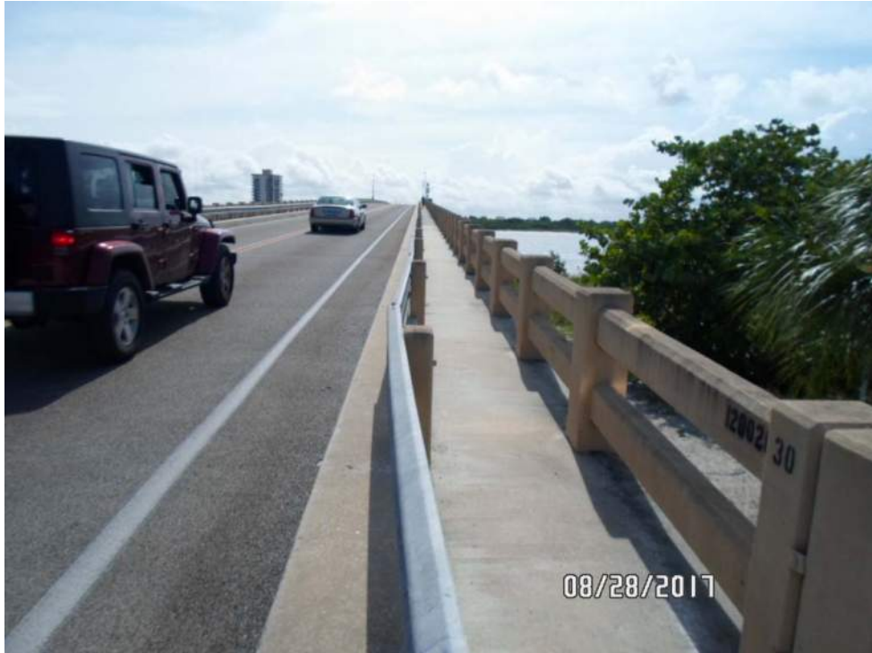
Homogeneous Area #11 (sample 031-033): Gray sidewalk concrete, west end of bridge looking east
