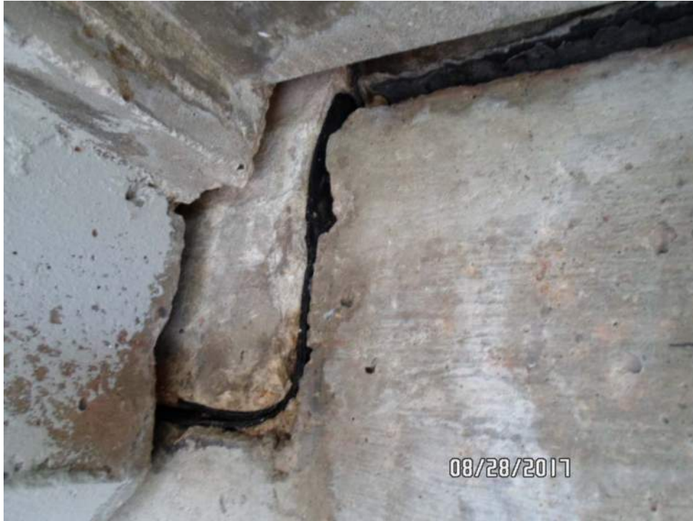
Homogeneous Area #7 (sample 019-021): Black felt pad- end bent between girder and end bent
