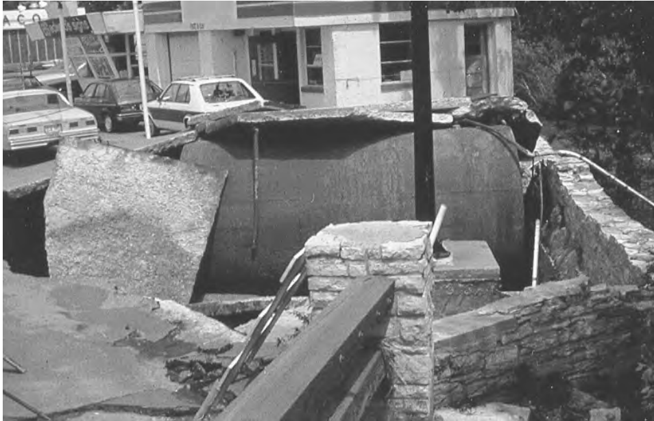
Figure 3.2.3.1A: Tank lifted by buoyancy forces
