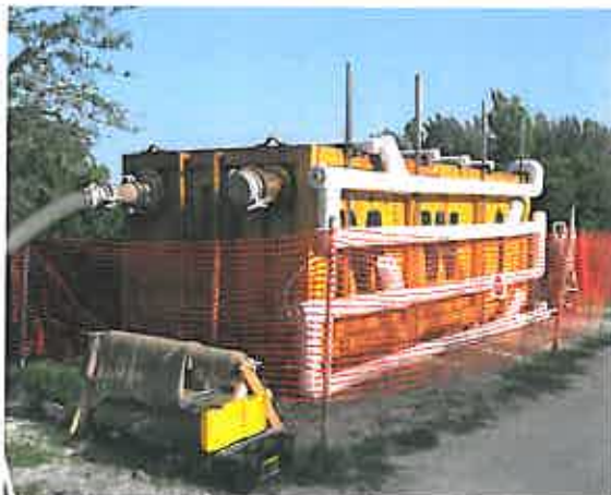
Photo 2: Pilot plant, outlet view.
