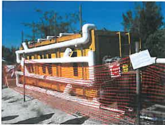
Photo 1: Pilot plant, inlet view.
