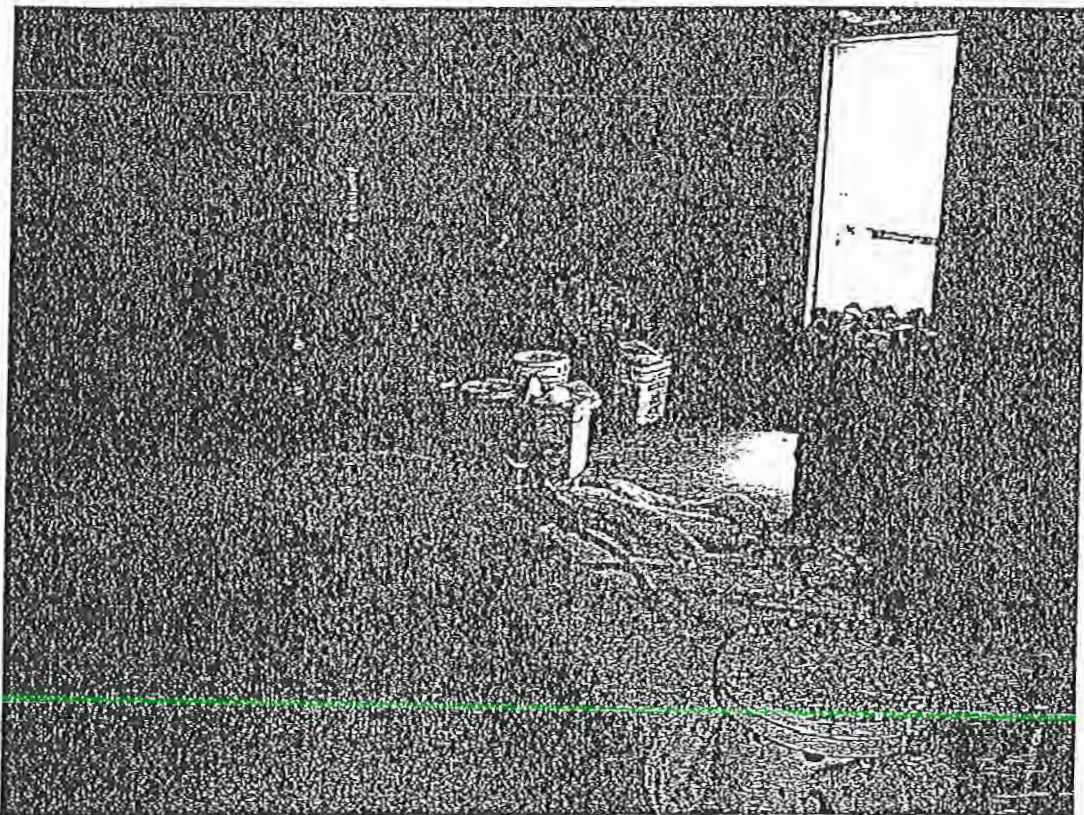
PHOTO 4 - WASTE OIL STORAGE IN FIRE SUPPRESSION PUMP HOUSE
