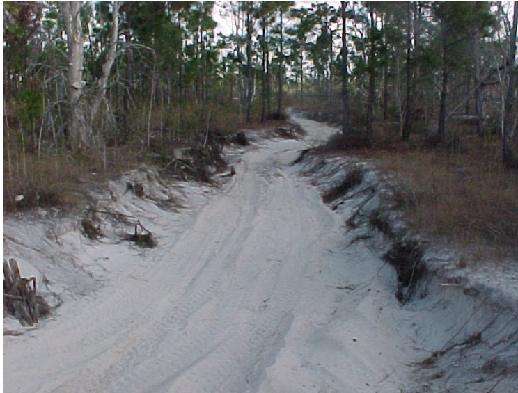
Vehicular Access Way East of Burnt Store Road Acting as a “Conveyance Channel”
