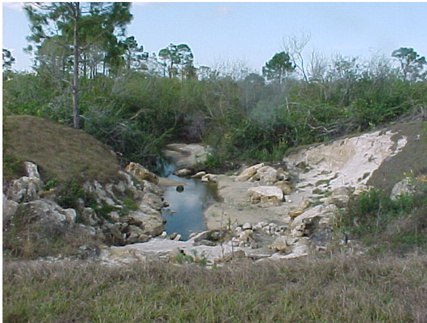
Culvert #5 – Failure of Bank on the Downstream Side
