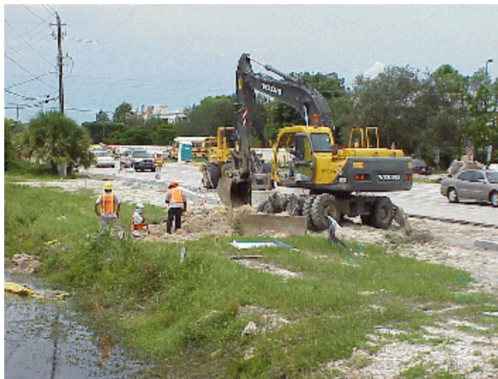
Widening of Cypress lake Drive from four lanes to six lanes west of U.S. 41.
