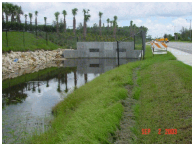
Storm water management control structure along the newly completed Three Oaks Parkway Extension south of Corkscrew Road.
