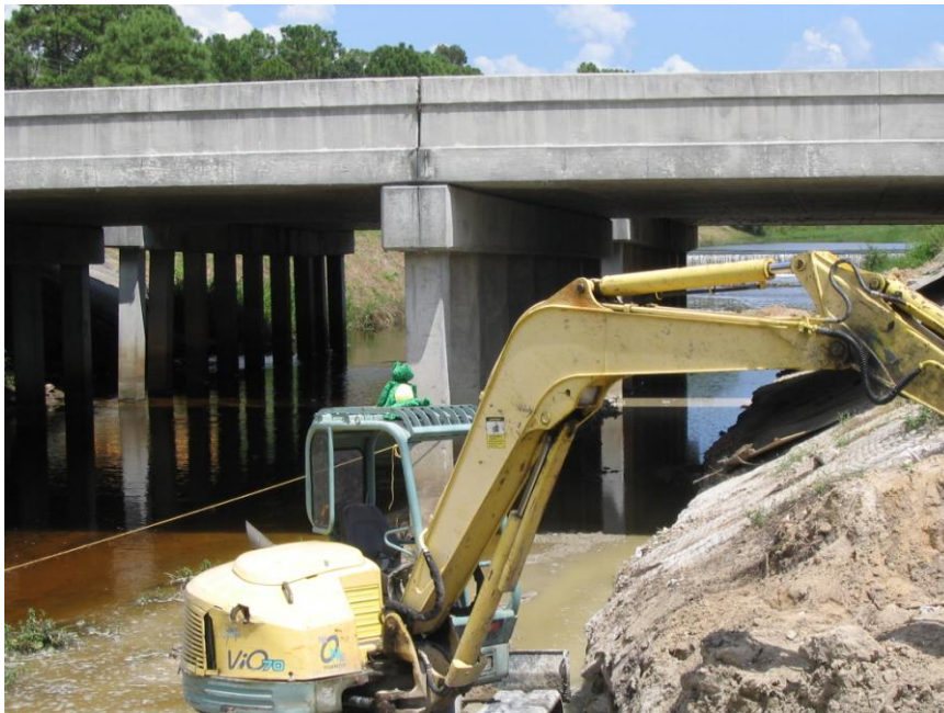
August 18, 2005 Preparation for excavation for pipe foundation. Looking north towards Daniels Parkway Bridge.
