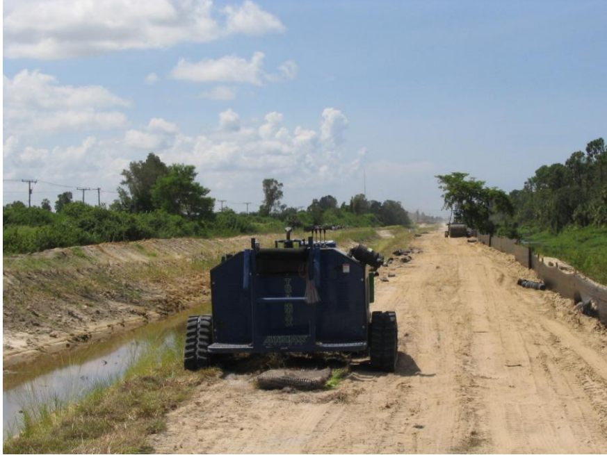
August 18, 2005 Cell No. 3 excavation complete. Sod laying operations on the berm Maintenance road between the filter marsh (to the left) and Ten Mile Canal (to the right).
