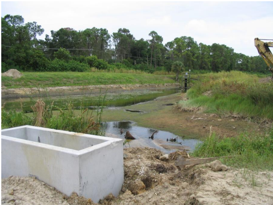
September 21, 2005 Controllable screw type sluice gates under construction. Looking northwest north of Daniels Parkway.
