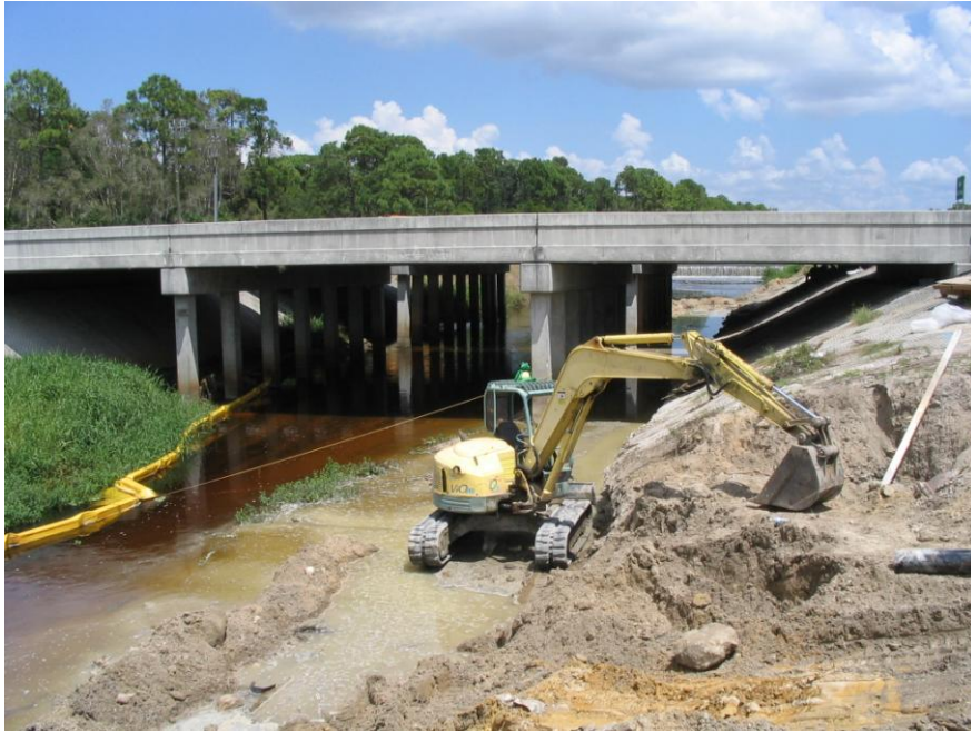
August 18, 2005 Turbidity control in the canal. A clear difference from canal water from turbid water around construction area. Looking north towards Daniels Parkway Bridge.
