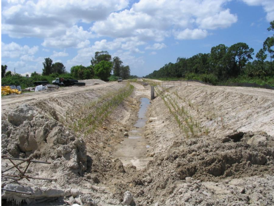
August 17, 2005 First Cell looking south with over flow riser to the west. Note side slope plantings of spartina bakeri. (sand cordgrass)
