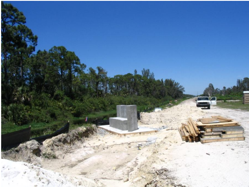
April 4, 2005 The bridge foundation on the east side of the canal. Filter Marsh site to the east of the canal prior to excavation. Looking north.
