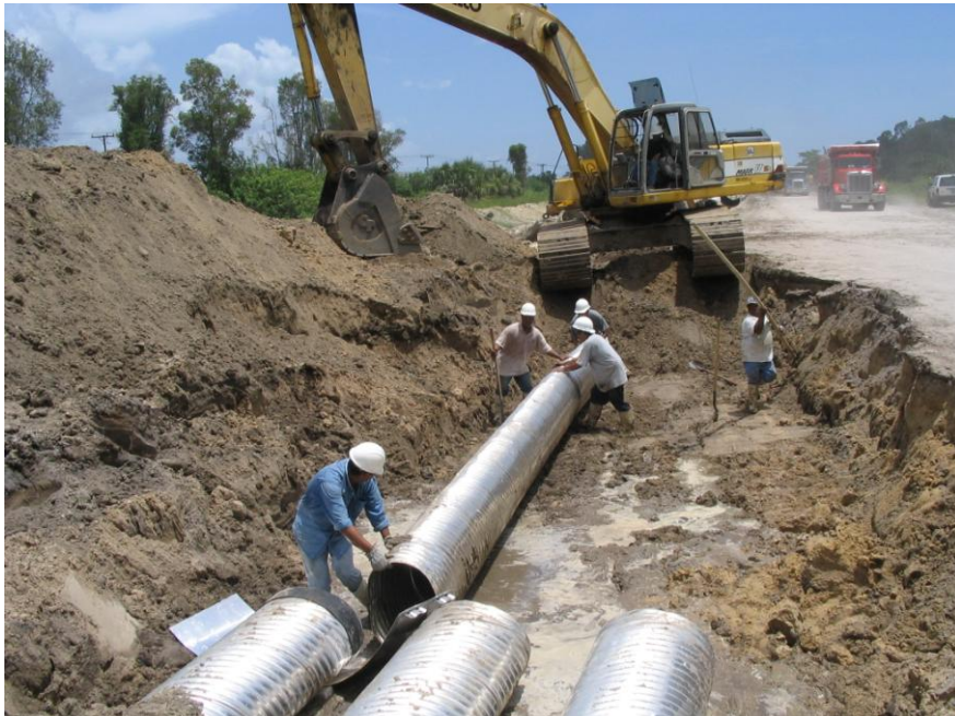
July 11, 2005 Laying pipes that convey water from one cell to the other. Looking south.
