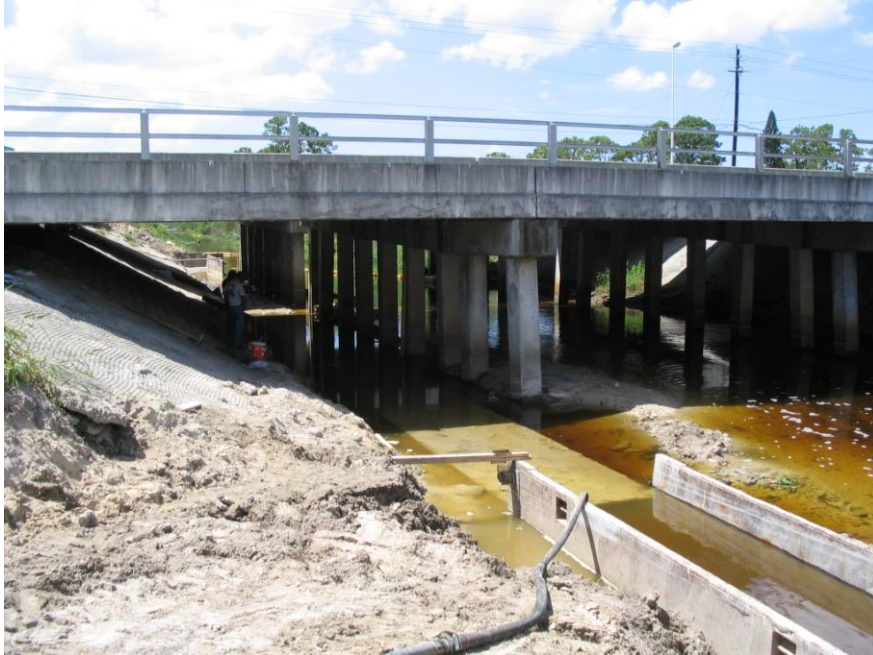
August 17, 2005 Foundation for two (2) 30-inch diameter pipes under the bridge, being constructed to support the pipe. Looking south under Daniels Parkway Bridge.
