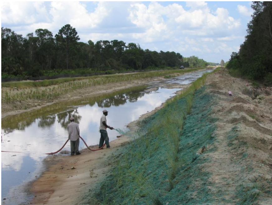
August 18, 2005 Solis stabilization and spartina bakeri (sand cordgrass) plantings along east bank of Cell No. 2.
