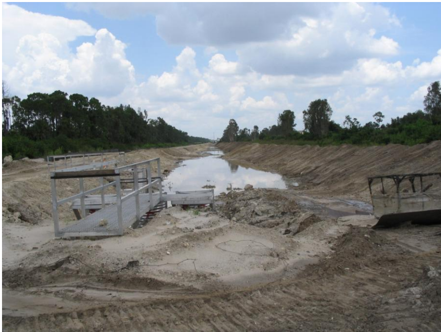
August 2, 2005 Cell No. 2 during construction. Maintenance access ramp is to the right. Looking north.
