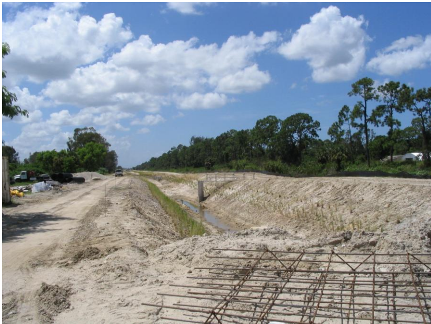
August 17, 2005 Settling basin to the south with over flow riser in the foreground, which discharges to the west into Ten Mile Canal.
