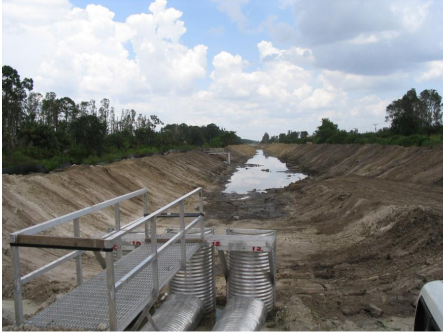
August 2, 2005 Cell No. 3 during construction. Maintenance access ramp is to the right. Looking north.
