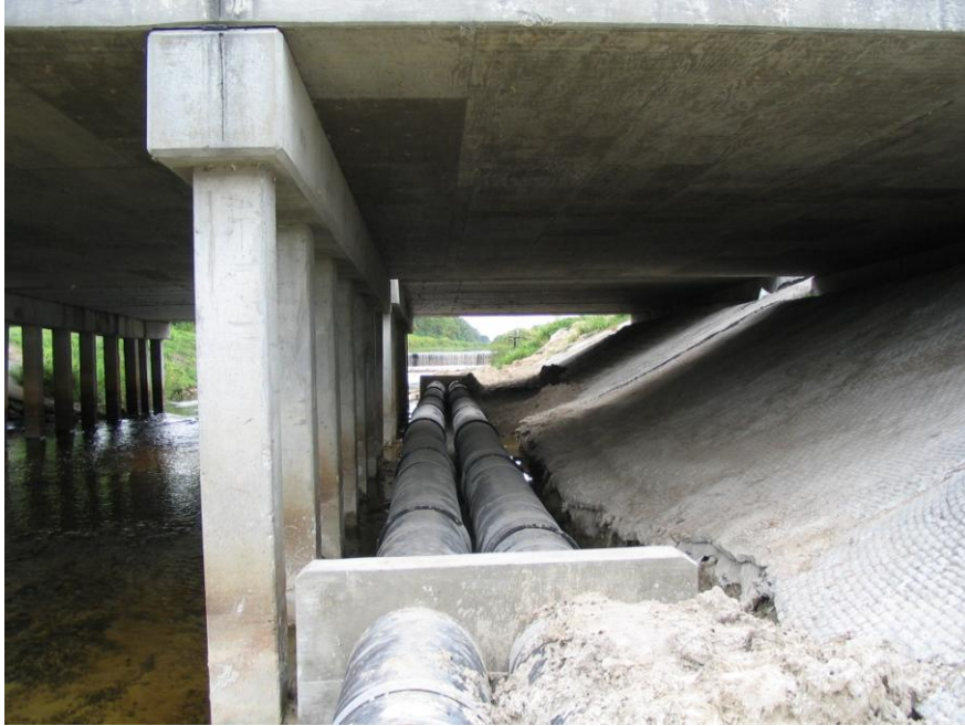
September 7, 2005 Construction of the two (2) 30-inch diameter cast iron steel pipes completed under the Daniels Parkway Bridge. Looking north.
