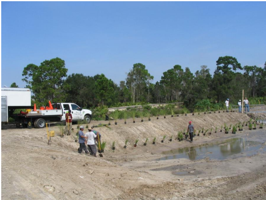
August 4, 2005 Side slopes of Cell No.4 under construction. Looking northwest From the south end of the filter marsh.
