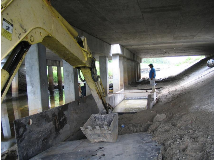
August 2, 2005 Preparing for laying foundation for pipes under the bridge. Looking north.
