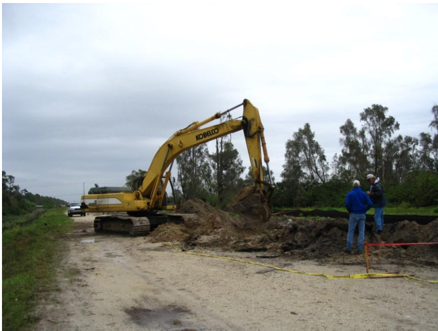
March 28, 2005 Excavation of filter marsh cells and discovery of buried debris. Looking north. Ten Mile Canal is to the left.
