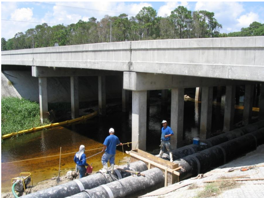
August 30, 2005 Preparing concrete forms to secure two (2) 30-inch diameter pipes on the foundation.
