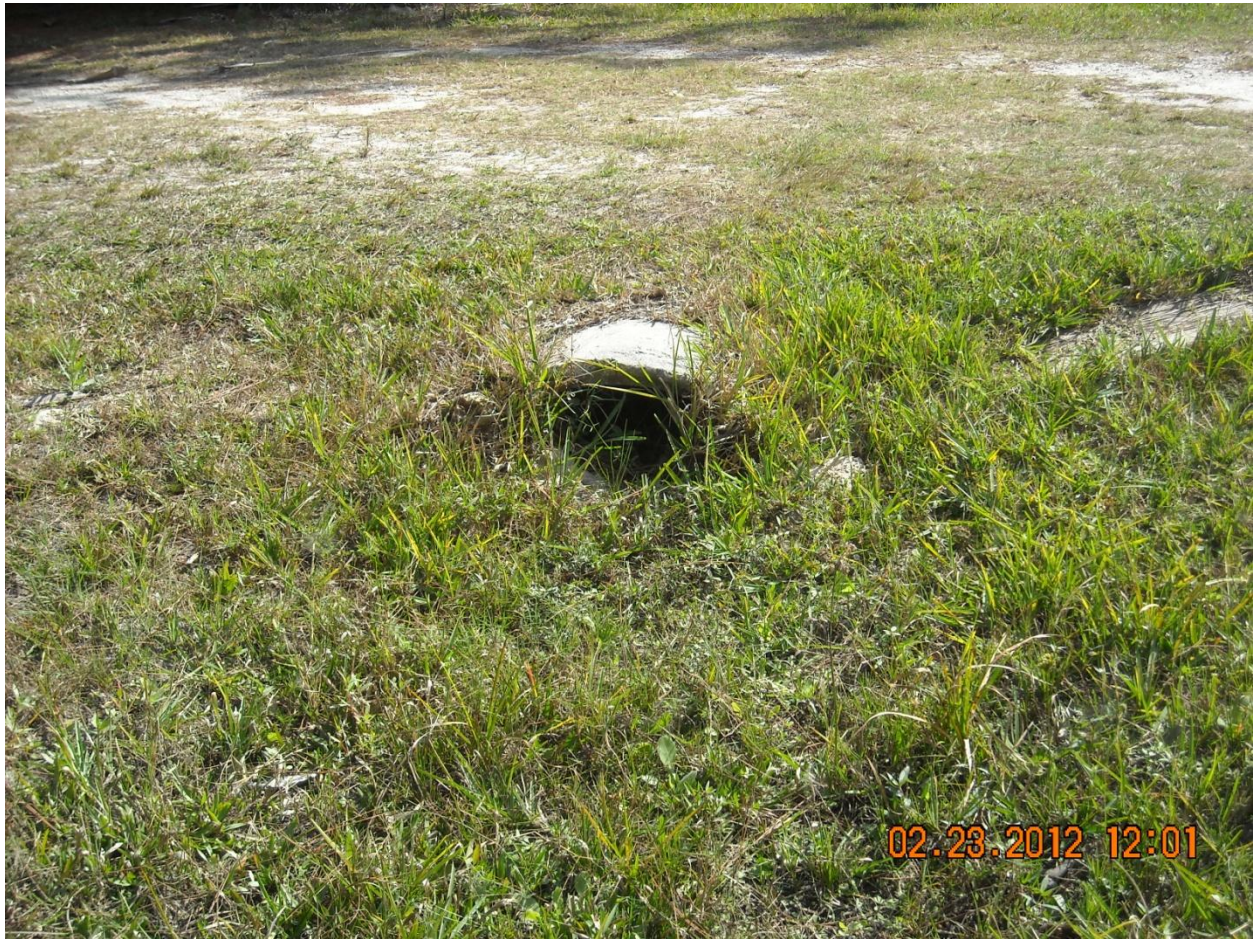
Poorly maintained culvert
